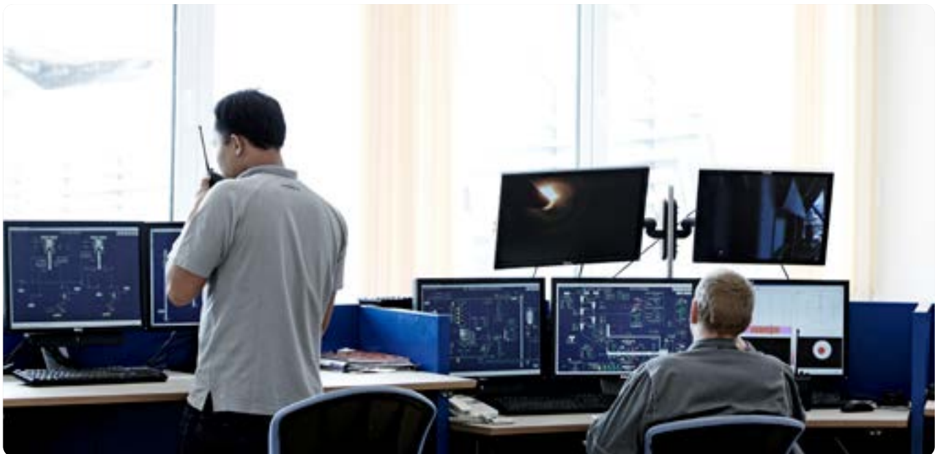
ECS Control Center
